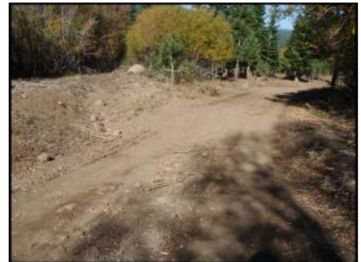
Photo 10b – Typical Existing Rolling Dip Needing Improvement
