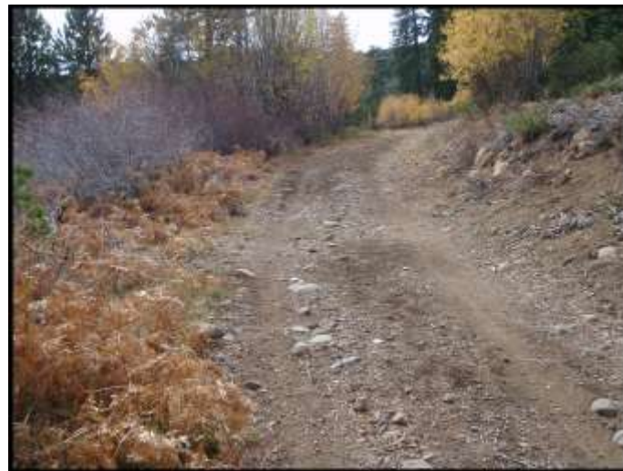
Photo 10e – End of Project Area Just West of Trailhead at Skislope Way
