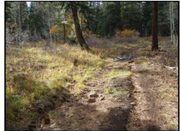
Photo 12b – Mid-Project Typical of Roadbed Degradation and Erosion
