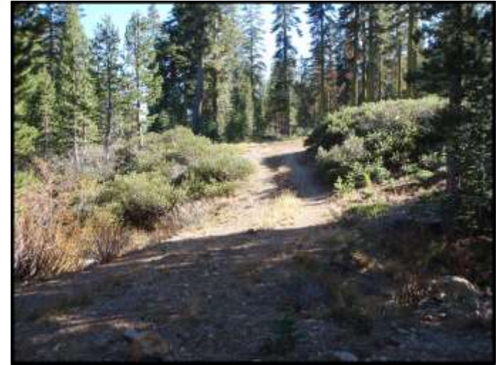
Photo 14c – North End of Trail Connection at Existing Dirt Road – Existing Culvert Crossing in Foreground
