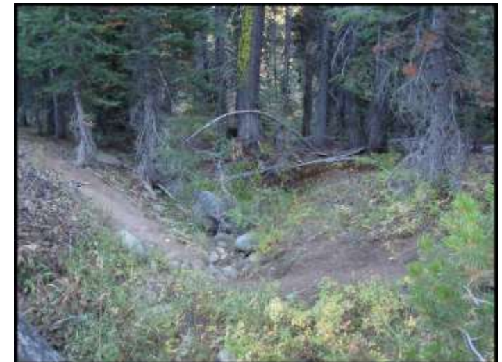
Photo 3d – Trail Crossing of Larger (<10 cfs design flow) Drainage Path / Perennial Drainage w/ Bridge
